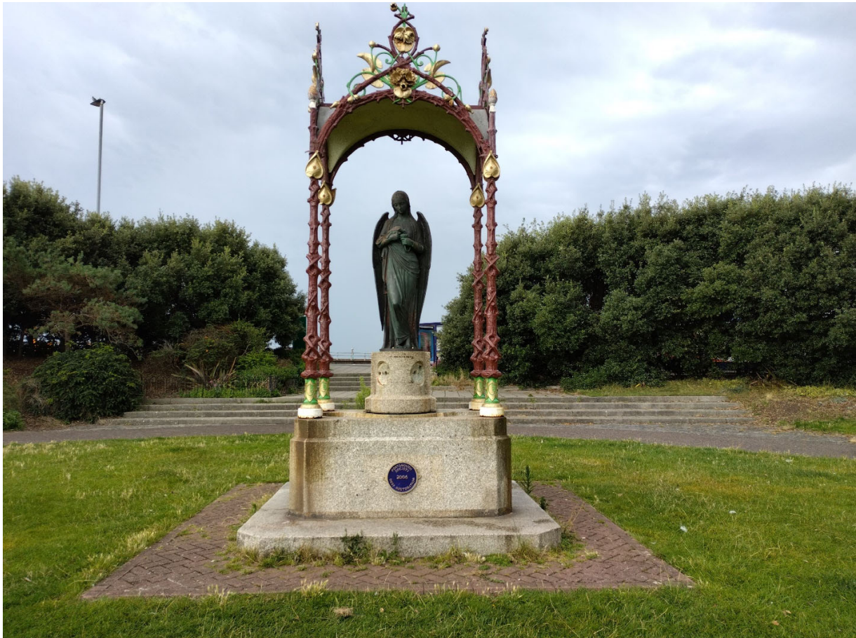
Photo showing weed growth in paving blocks at a base of the statue.
